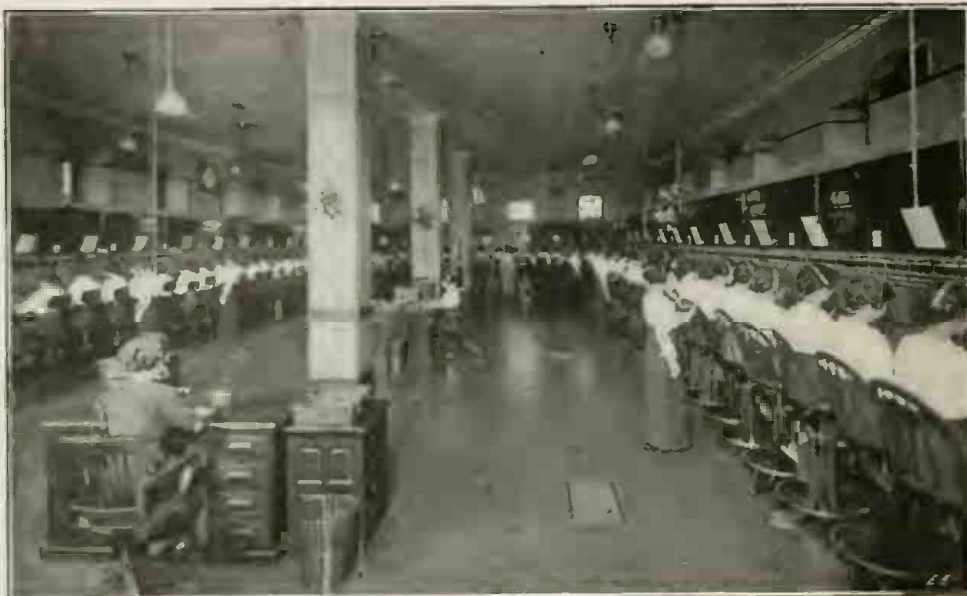
Fig. 4. Contrast This Picture of a Modern Telephone Exchange With Those of the First Telephone Switchboards Shown on the Preceding Page. Instead of Waiting Half-An-Hour For a Call, It Is Now Put Thru in 10 Seconds.
